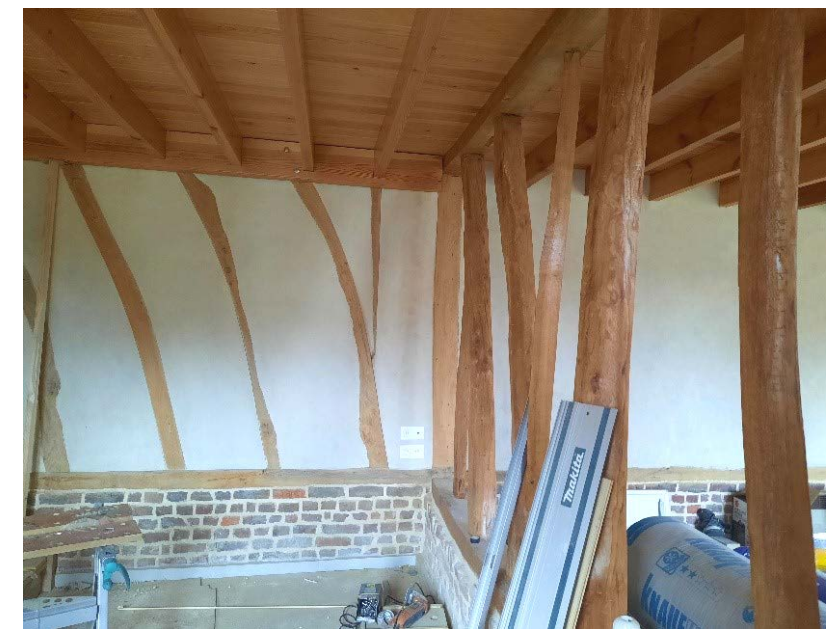
Inside, the dwarf wall is made of brick, with a stringer on top supporting the wooden frame (photograph by Mathilde Duval, coll. CHHP 2022).
