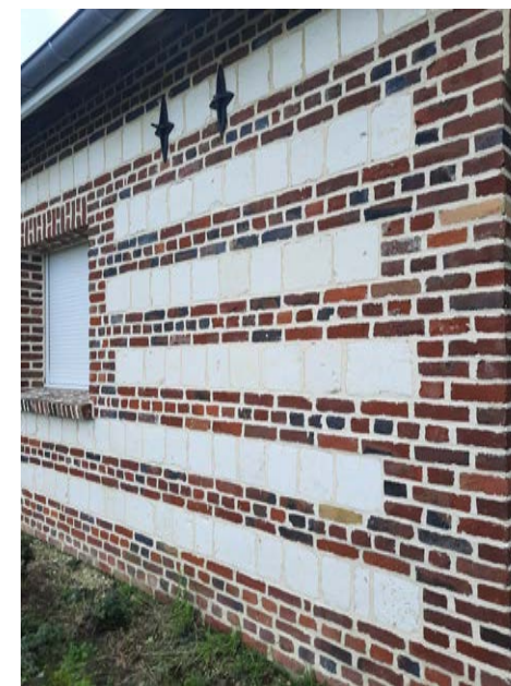
A rouge-barre wall at the back of this cob-built house has been renovated: this brick-laying technique alternates a row of stone with three rows of brick (photograph by Mathilde Duval, coll. CHHP 2022).
